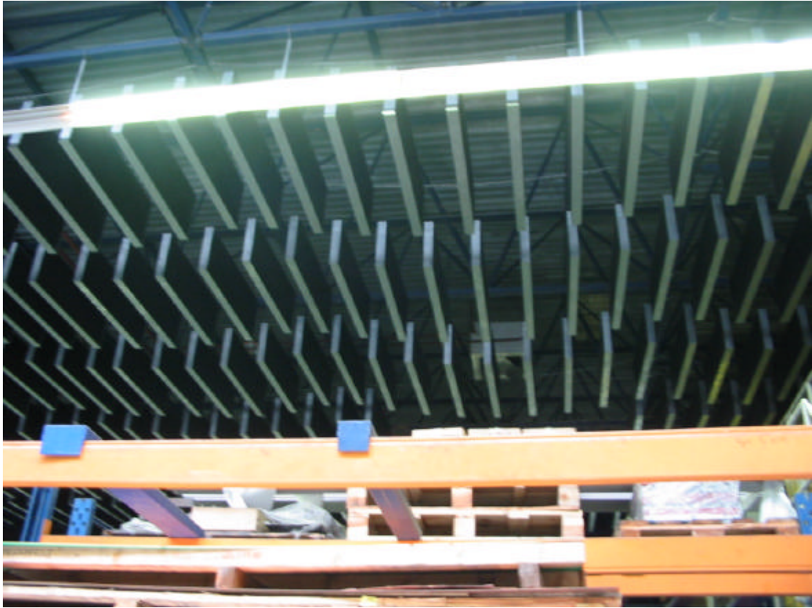
Figure 3: Sound absorbing baffles under roof
