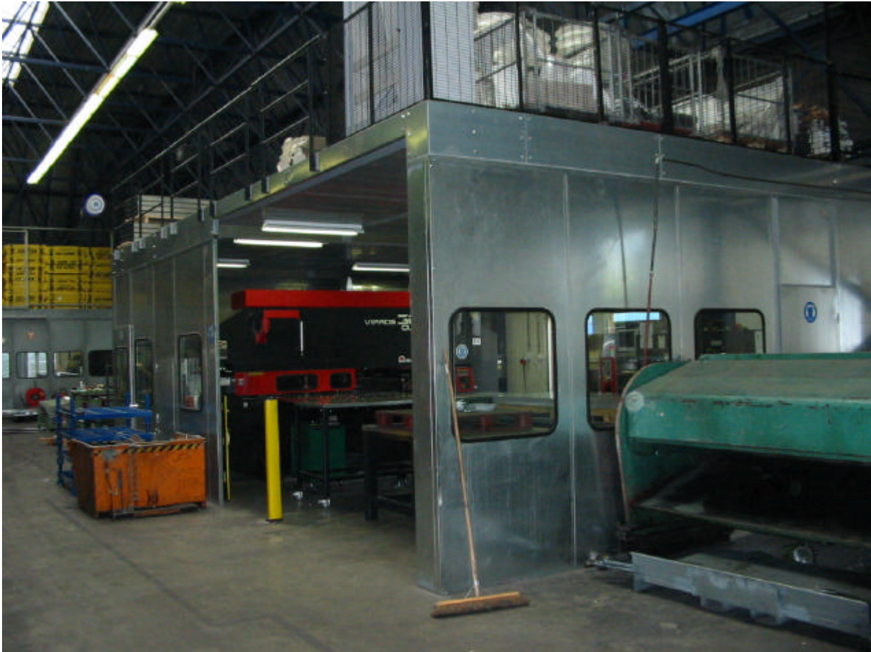
Figure 2: Sound insulating enclosure around punching machine
